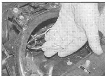
13.7 Rear turn signal wiring connectors – XL650V
