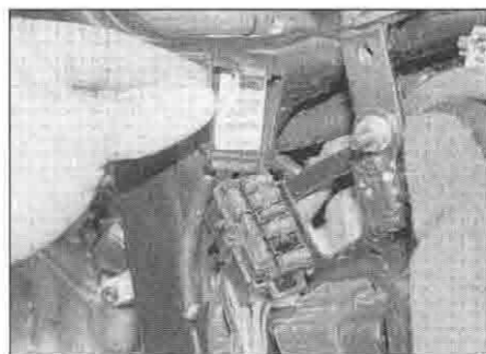
5.3e ... to access the fuses
